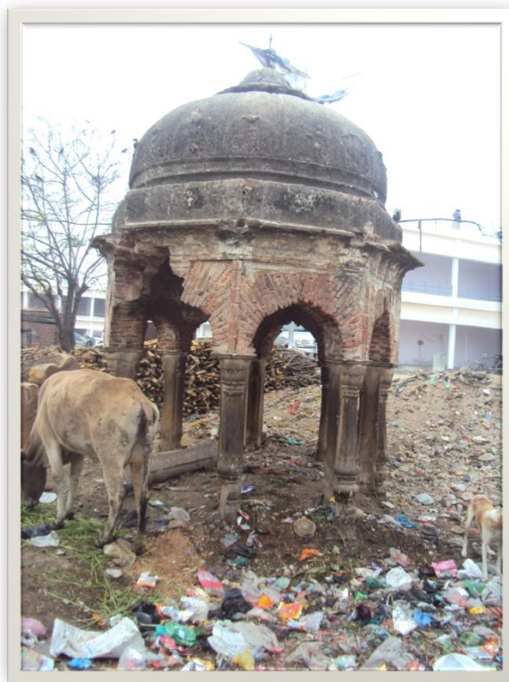
Canopy Before Repair
