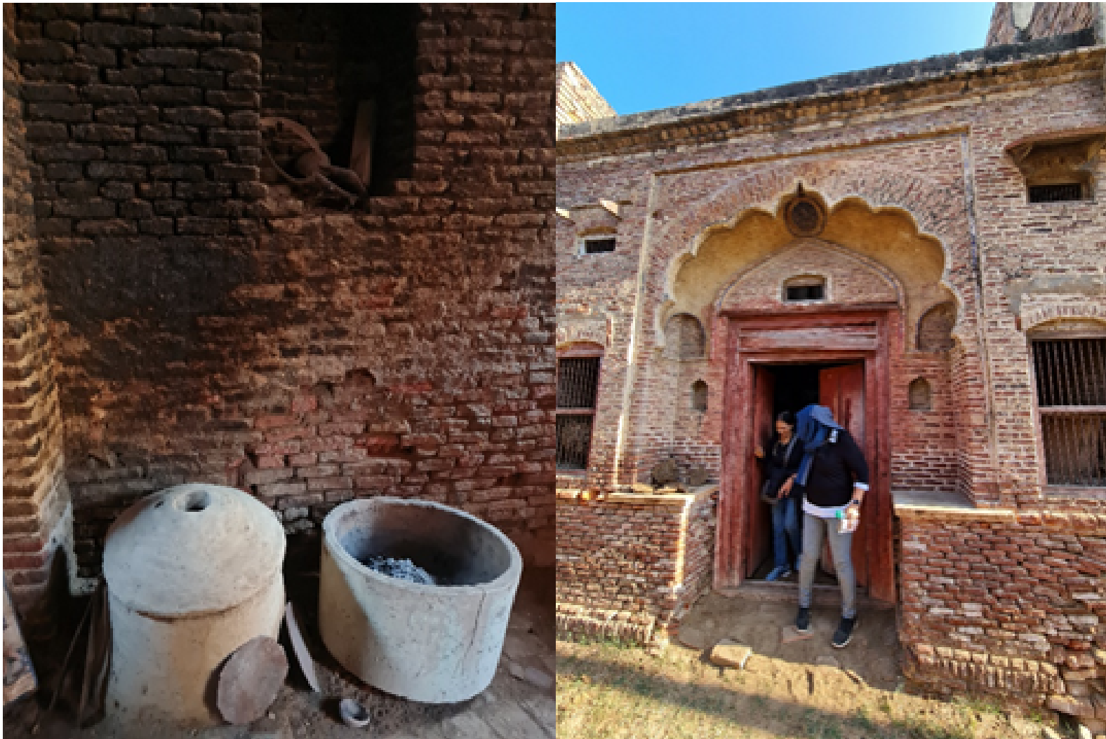
Fig 5-6: Inside the 19th century Haveli a keep warm 'oven' that ran with heated terracotta balls, The exterior of the Haveli showing an ornate yet exposed brick multifoliate arched entrance; Ms. Tapasya Samal
