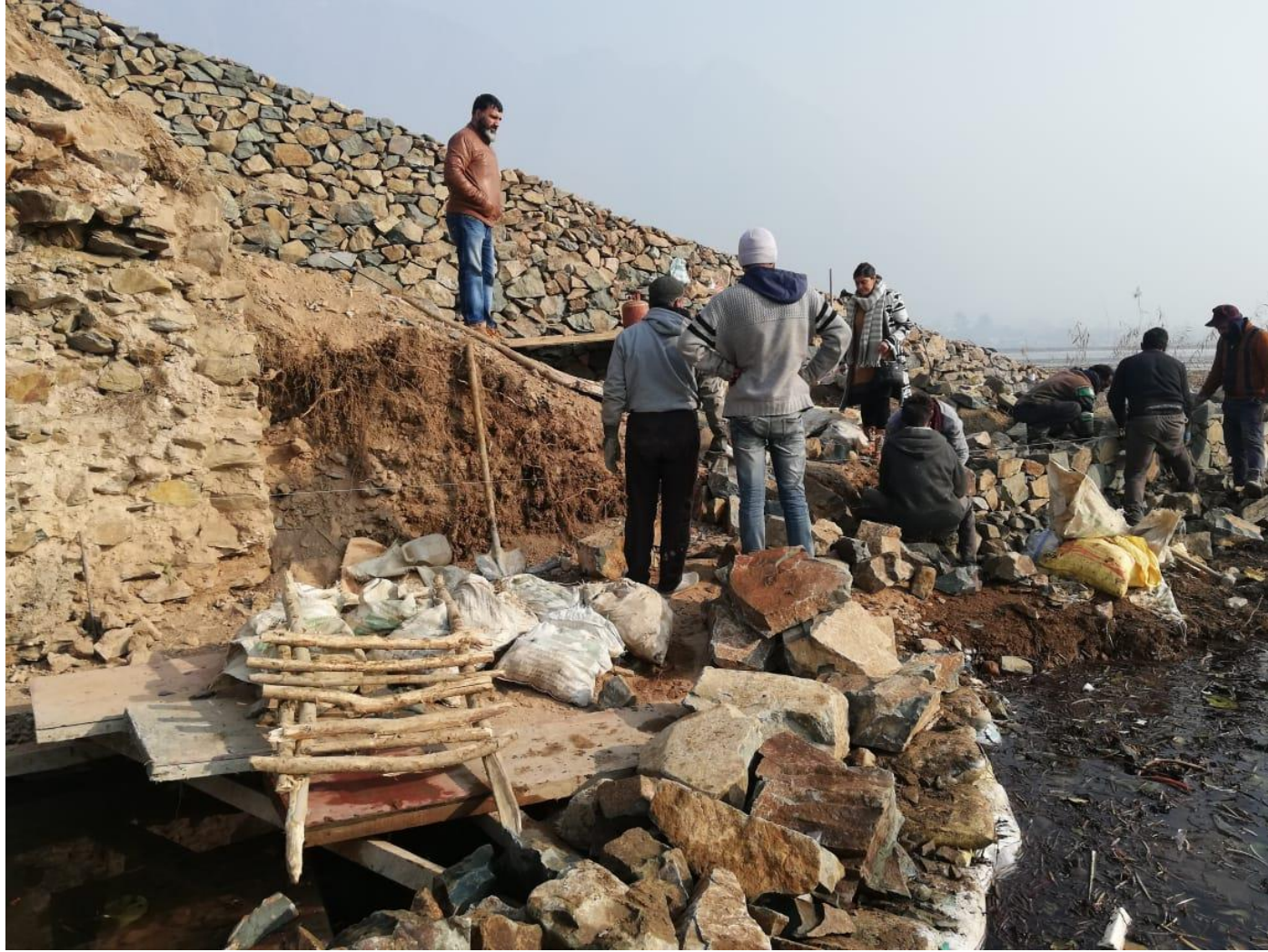
Photo: Ongoing restoration of historic OontKadal in Dal Lake, Srinagar © INTACH, J&K 2019
